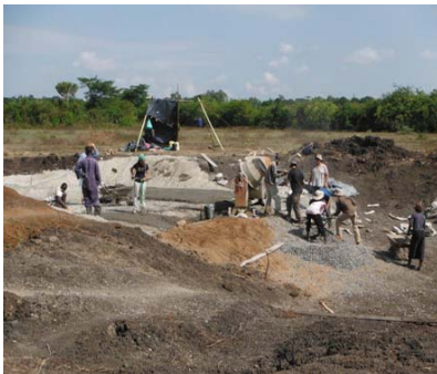
Construction is underway to install a concrete spillway on the local dam
