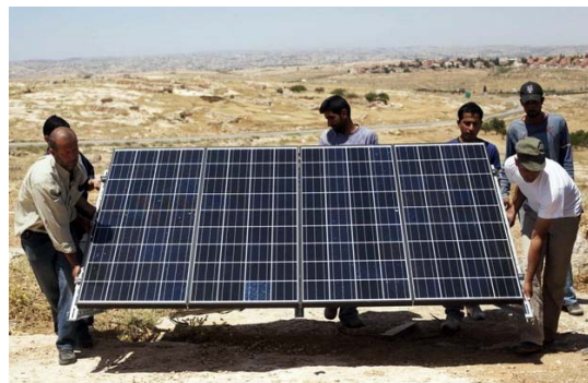
Solar power project Israel
